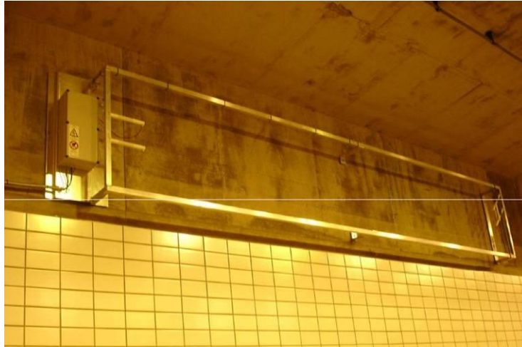
Figure 10: Fine dust reduction system installed in the Thomassentunnel (Delft University of Technology and BAM, 2009).
